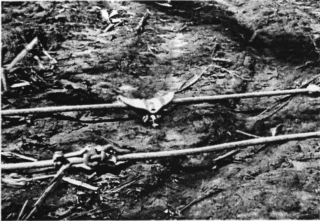
Fig. 1-6 (a) : Conductor after separation from insulator
